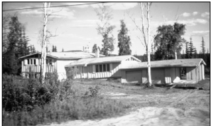
This house was built on ice-rich permafrost. Heat from the house caused the permafrost to thaw and the ground surface to settle unevenly resulting in bending and twisting of the structure which was ultimately abandoned (photograph by Tom Osterkamp).
