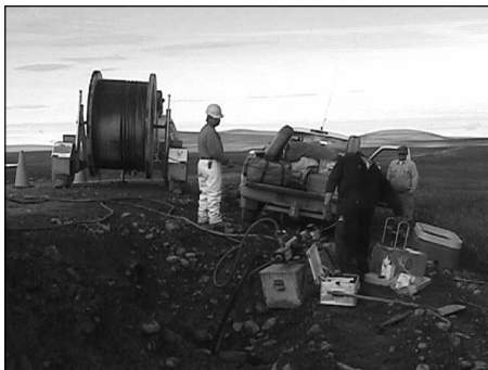
Fiber-optic cable has been brought in to Toolik Field Station; design and installation of the local area network will be completed in Summer 2000. The fiber-optic line replaces the VHF radio/microwave-based telephone communication system that has served the labs since the early 1990s. This upgrade became possible when Kanas Telecom, Inc. completed installation of a fiber-optic line paralleling the Trans-Alaska Pipeline from Prudhoe Bay to Valdez (photo by Mike Abels).
